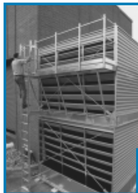
External platform at louver face
