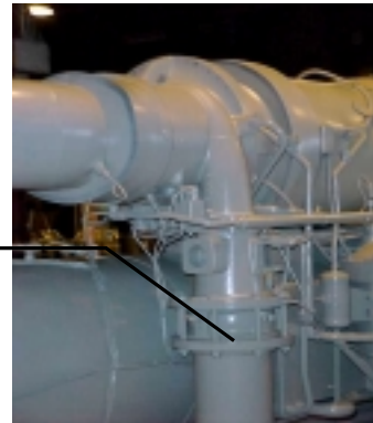
Discharge line check valve combines with main liquid shutoff valve to isolate the condenser
