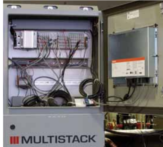
Example of Master Control Panel hardware with defined inputs and outputs for a two compressor system.
