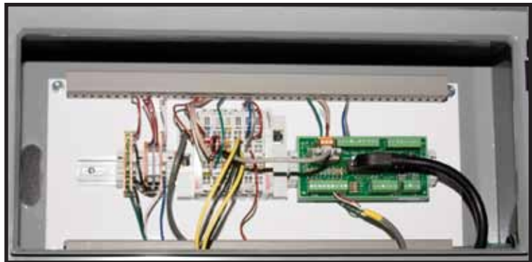
Example of a typical Compressor Hub hardware layout with defined inputs and outputs.
